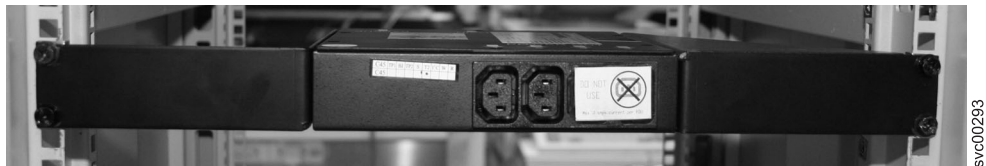
Figure 7. Positioned in rack
